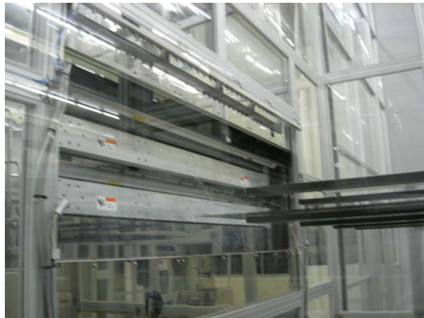
Figure 7. Ionizer installed at load area and robot arm deliver glass panel 5m/sec.
